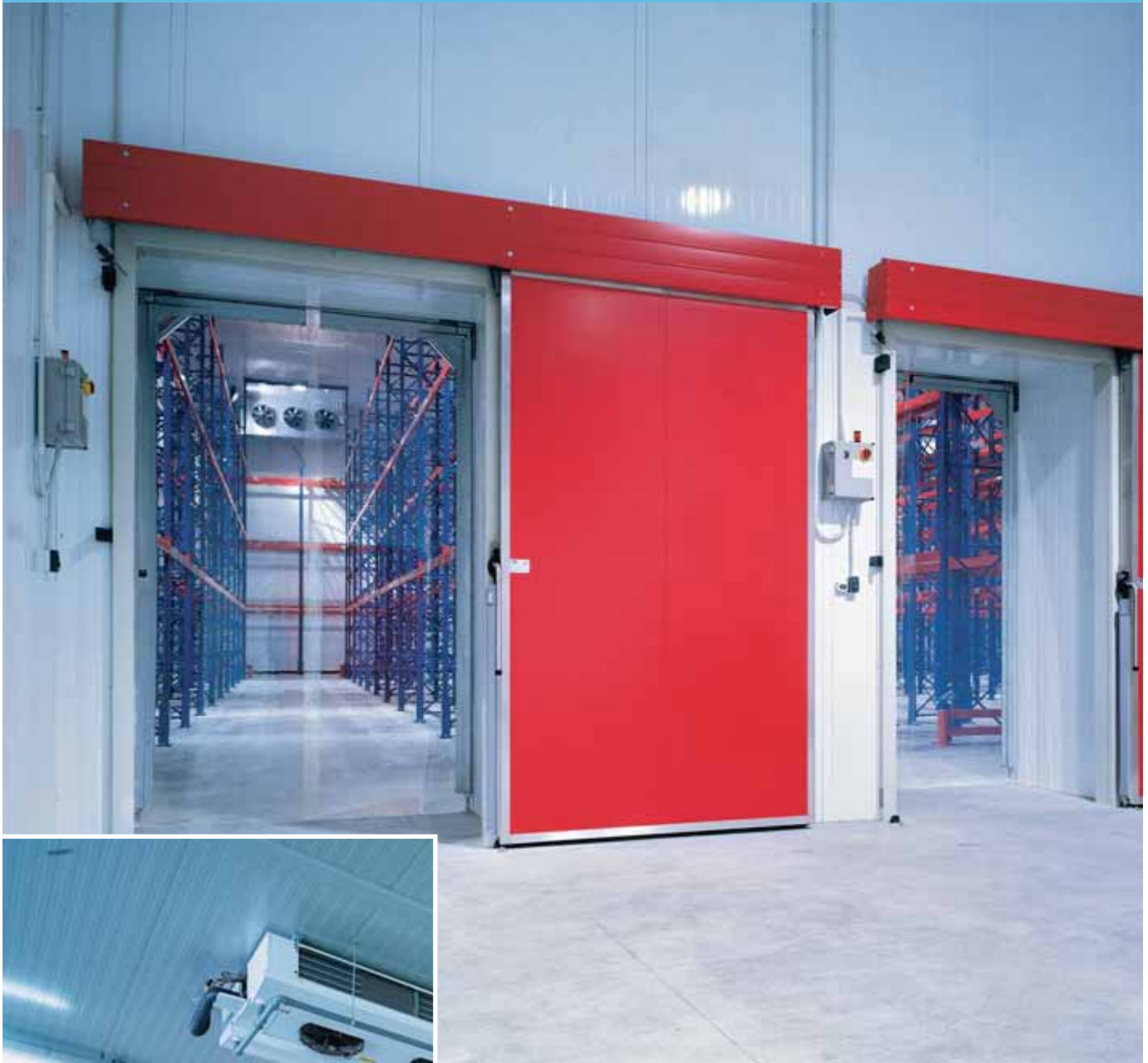
Cold rooms in Verona
